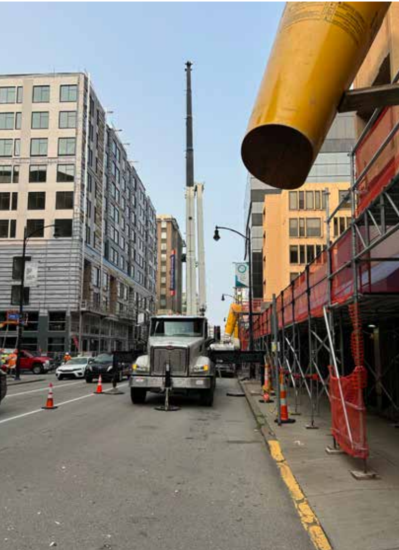
Construction on Forbes Avenue requires major traffic control and staging on one of Pittsburgh's busiest streets. Photo by Catherine Donahue.
